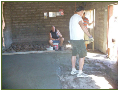
Constructing cement floors – keeps the children from living on mud which can cause worms and other issues
